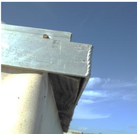
Incorrect measurement will create a gap between the curb and the skylight frame
